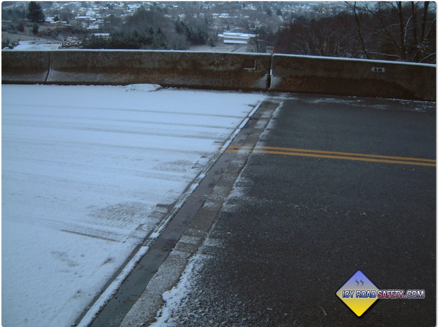
Fig 3e: Icy bridge road surface condition transition zone
