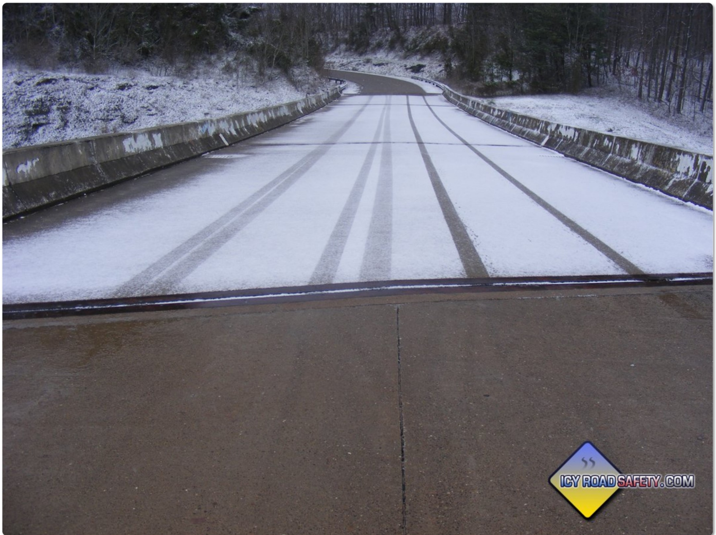
Fig 3c: Icy bridge in Kanawha County, West Virginia
